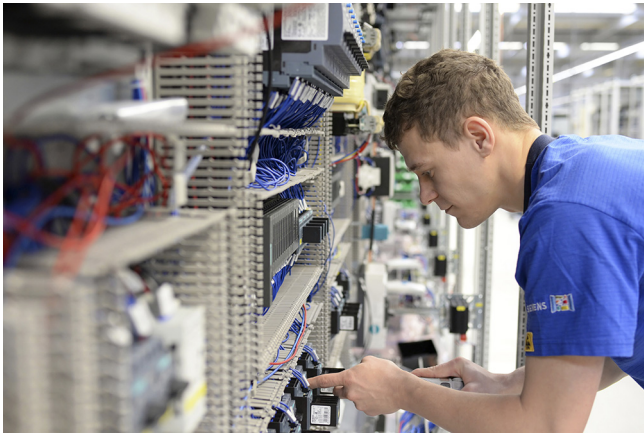
WKC - Control cabinet wiring
