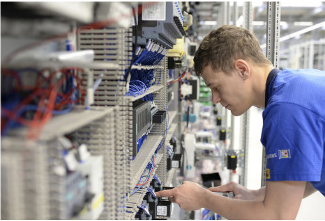
WKC - Control cabinet wiring
