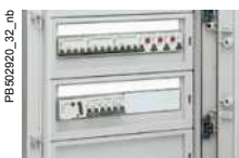
Detail from the Circuit Marking System
