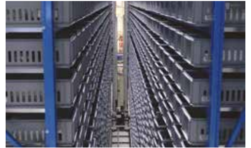
Rail dependent storage and retrieval equipment
